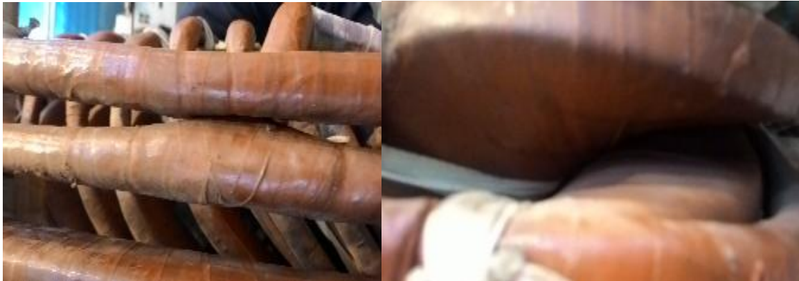
Fig. 2 : Low Clearance between Adjacent Phase Bus Connection
