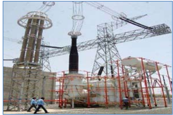
Figure 1(b): 1200 kV Multi-column surge arrestors
