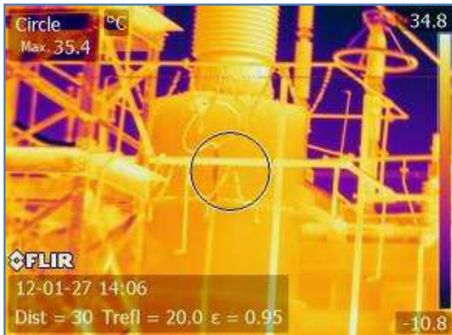
Fig. 8(a) : Thermograph image of bushing turret of transformer
