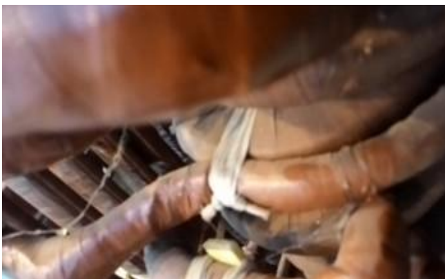
Fig. 3 : Wrinkle can be Seen in Overhang Connections
