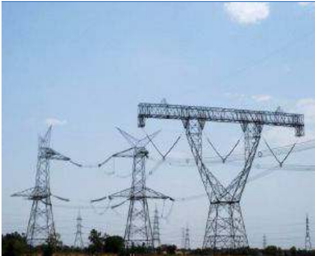
Fig. 3(a) : 1200kV Single circuit test line (S/C tower height: 55 m)
