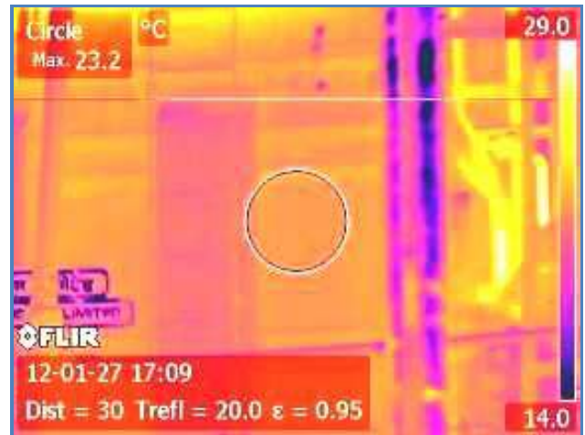
Fig. 8(b) : Thermograph image of the transformer body
